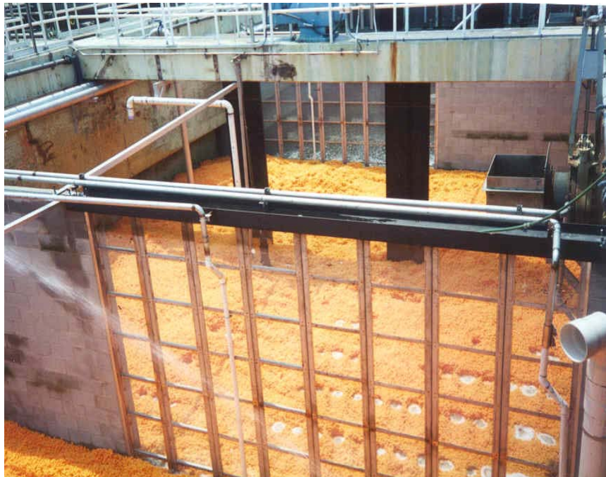
Media installed in aeration basin with screens on either side to retain the media.
