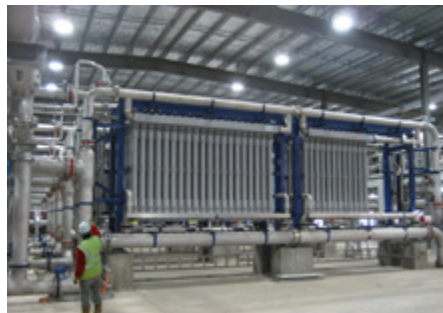
Figure 11. MEMCOR CP at Changi NEWater plant in, Singapore (Courtesy of Siemens Water Technologies)
