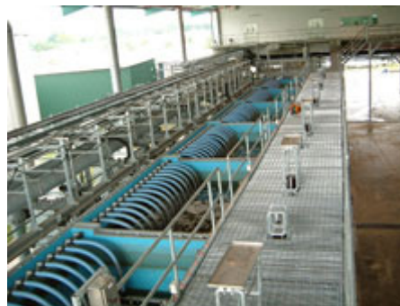
Figure 8 MEMCOR CS at Kranji NEWater Reclamation Plant, Singapore (Courtesy of Siemens Water Technologies)
